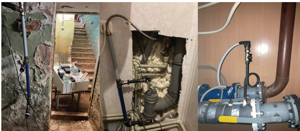
Figure 2. Measurements on a section of the water supply network
