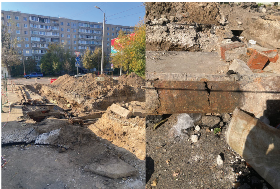
Figure 5. Pipe break in a section of the water supply network, Murom
